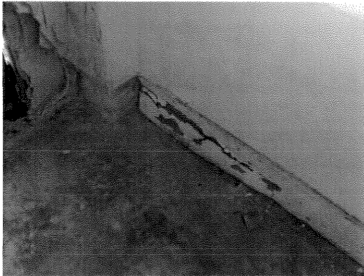
Typical unit rotted baseboard.
