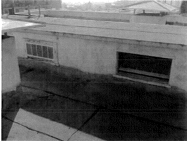
Elevator over ride at roof
