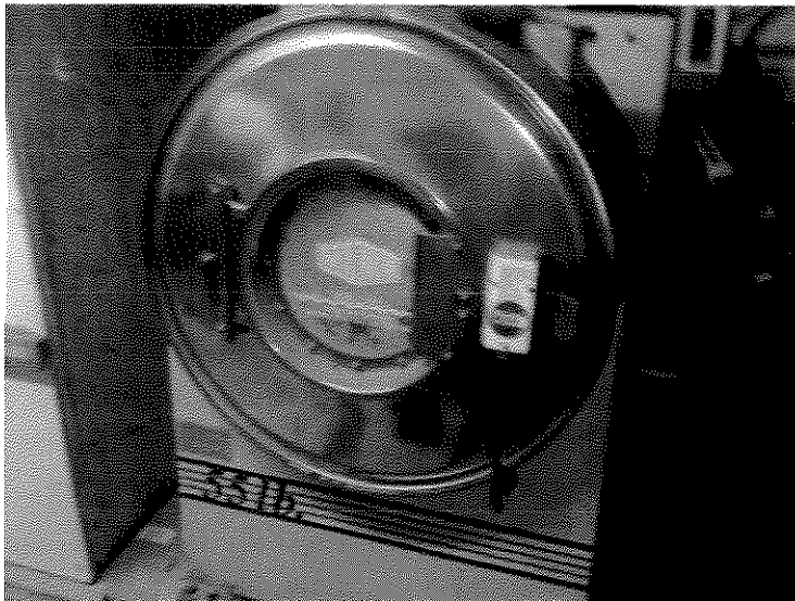
Existing commercial washing machine in basement.
