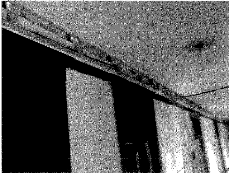
Typical soffit in corridors for electric wiring.
