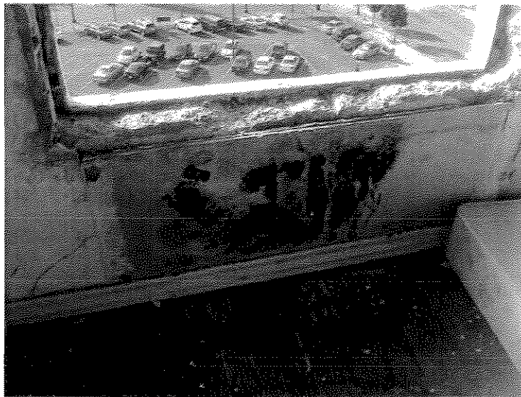
Mold on drywall at exterior wall.
