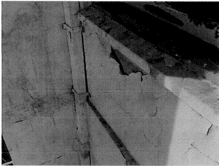
Exterior elevation showing peeling paint/stucco.
