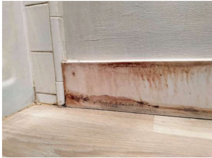
[PHOTO: Current condition showing severe water damage and mold on wooden baseboards near tub]
