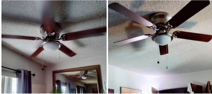
[PHOTO: Replacement ceiling fans installed by ██████████]
