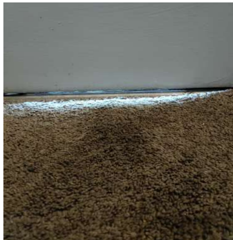
[PHOTO: Gap between door and carpet threshold, Nov 4, 2021]
