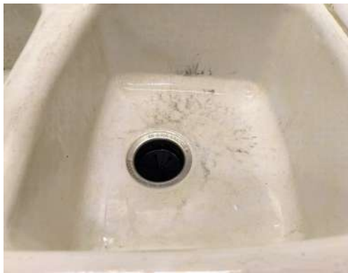
[PHOTO: Right basin showing extensive enamel degradation, Feb 14, 2026]
