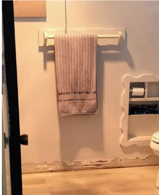
[PHOTO: Wall exposed during installation showing deteriorated drywall with water damage and mold]
