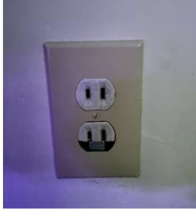
[PHOTO: Ungrounded two-prong outlet before replacement]
