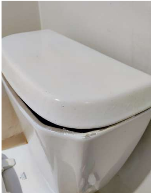
[PHOTO: Toilet tank with mismatched cover, Feb 15, 2026]
