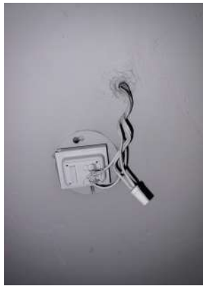
[PHOTO: Exposed electrical wiring - hallway closet ceiling junction box]
