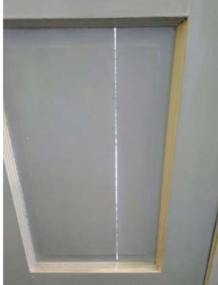
[PHOTO: Door crack running full length of panel, Nov 4, 2021]
