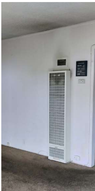
[PHOTO: Carpet near furnace area showing concentrated contamination May 28, 2024]
