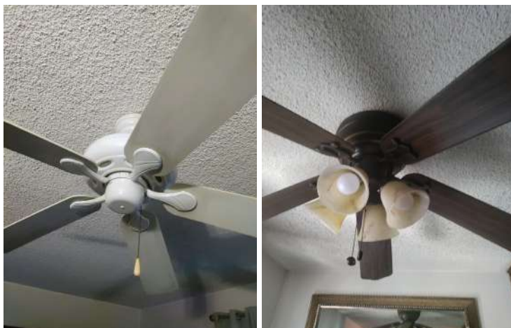
[PHOTO: Original ceiling fans before replacement]
