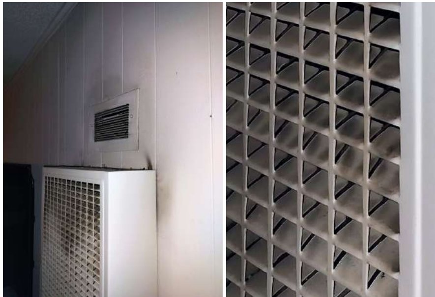
[PHOTO: Furnace Wall and grate showing heavy black soot Feb 2026]
