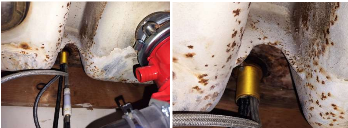
[PHOTO: Sink underside showing extensive rust corrosion, Feb 12, 2026]
