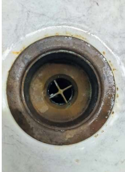
[PHOTO: Drain area showing severe rust corrosion, Feb 14, 2026]
