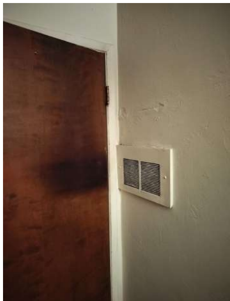
[PHOTO: Bedroom door and sealed vent showing soot Feb 2026]
