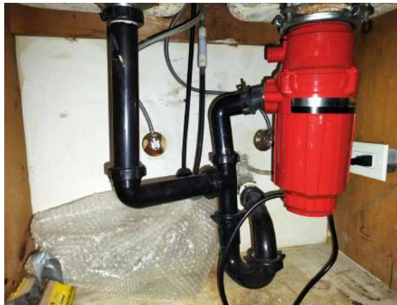
[PHOTO: Under-sink plumbing showing bubble wrap I installed per [REDACTED]'s directive, Feb 12, 2026]
