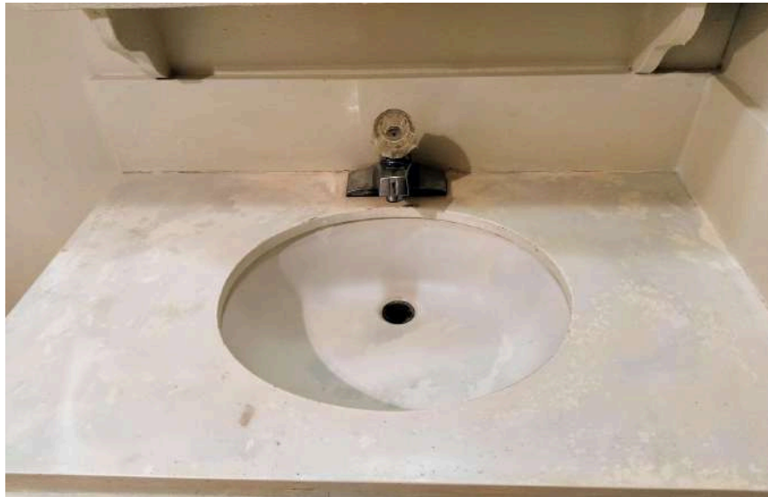
[PHOTO: Bathroom vanity current condition showing severe surface deterioration]
