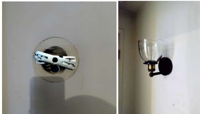
[PHOTO: Hallway wall sconce installed without switch]
