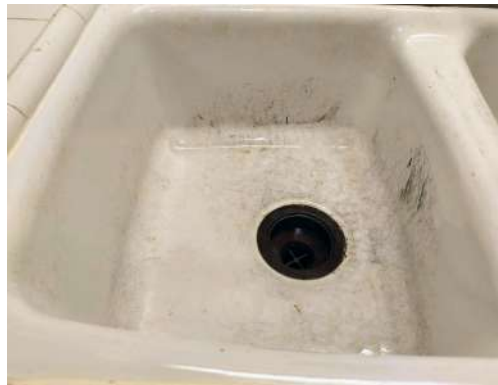
[PHOTO: Left basin showing extensive enamel degradation, Feb 14, 2026]
