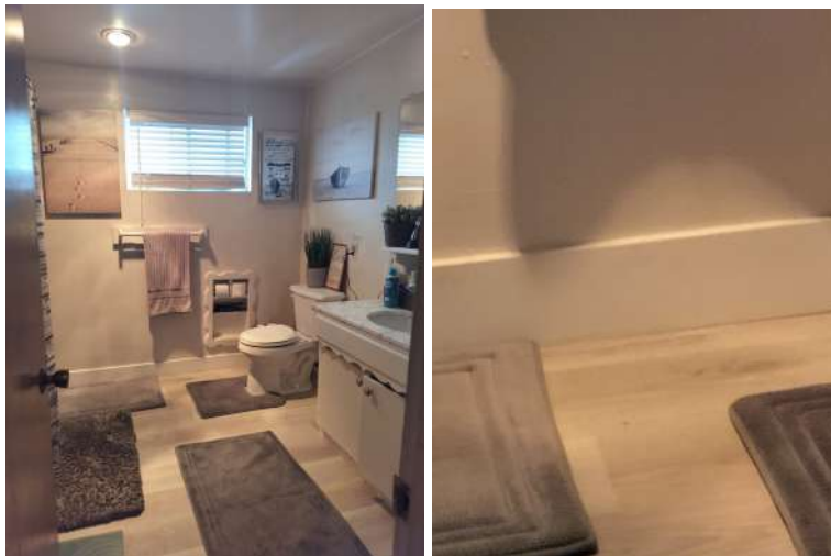
[PHOTO: Bathroom after installation with new vinyl and wooden baseboards concealing damage]
