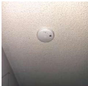
[PHOTO: Smoke detector installed in living room after October 2025 SDHC citation]
