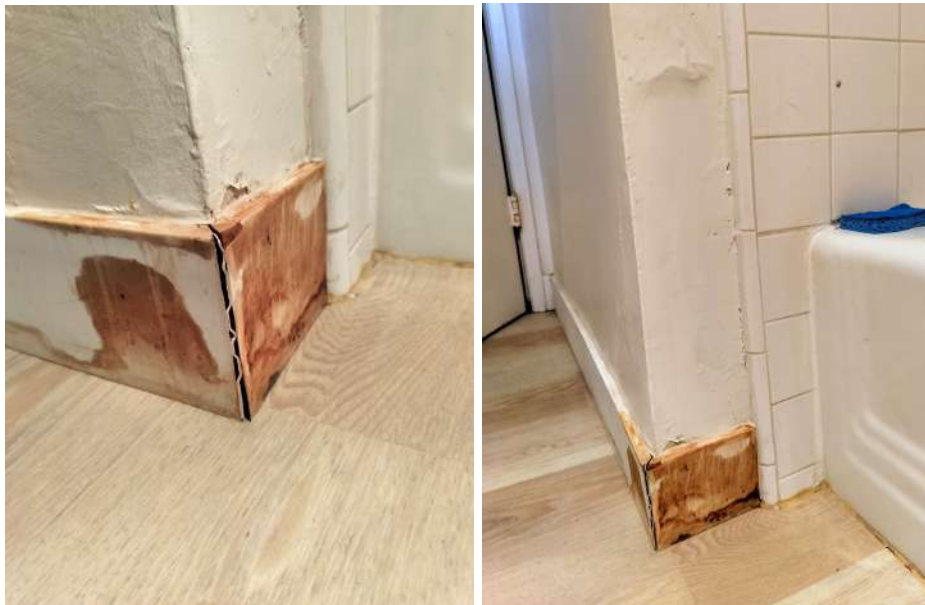
[PHOTOS: Corner near tub showing wooden baseboards separating at joint, saturated with moisture]
